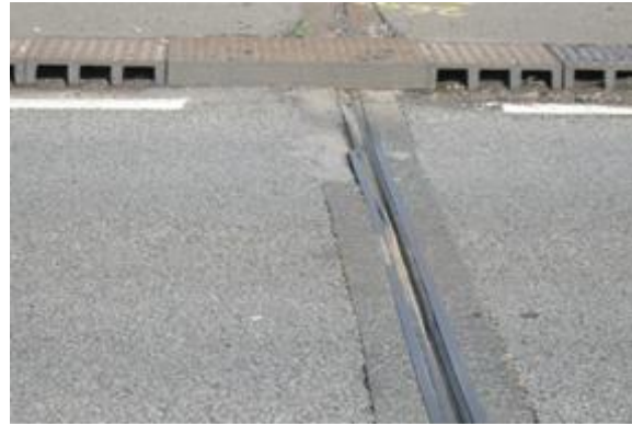
Bridge deck joint which has become dislodged and is an imminent hazard
