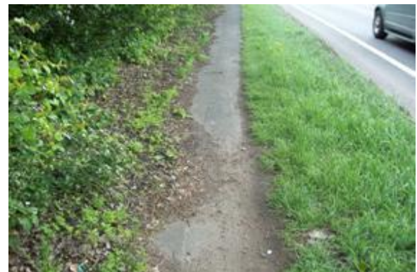
Trip hazards have a step change >25mm
