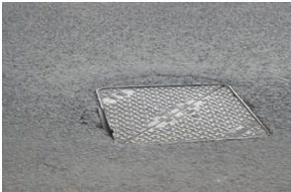
Hazardous example of difference in level around ironwork >25mm in trafficked areas
