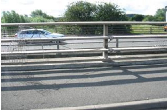
Parapet mesh missing, allowing direct access to carriageway from footway.
