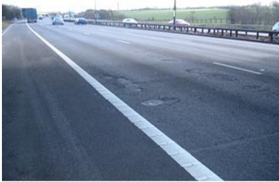
Hazardous example of paved area failure within trafficked area resulting in potholes >150mm or of a greater depth than the surface course thickness or >40mm depth.
