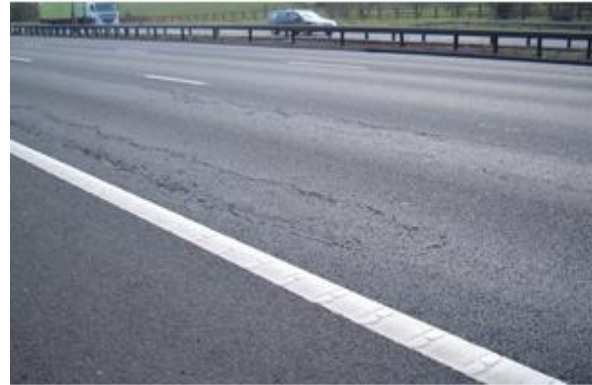
Hazardous example of a paved area failure in trafficked area with a deformation >40mm
