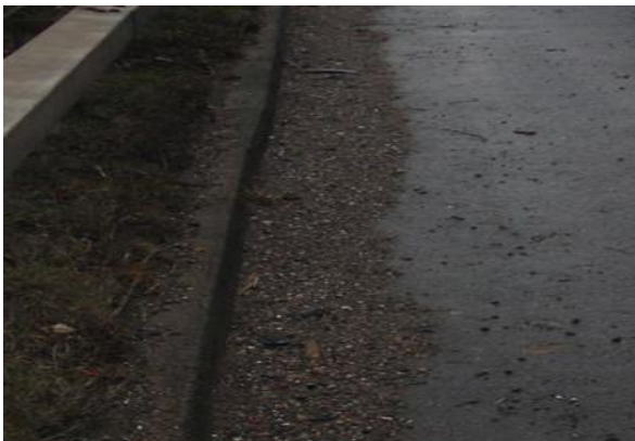
Excessive silt build up in channels can prevent surface water reaching outfalls and also presents a risk of skidding to motorists.
